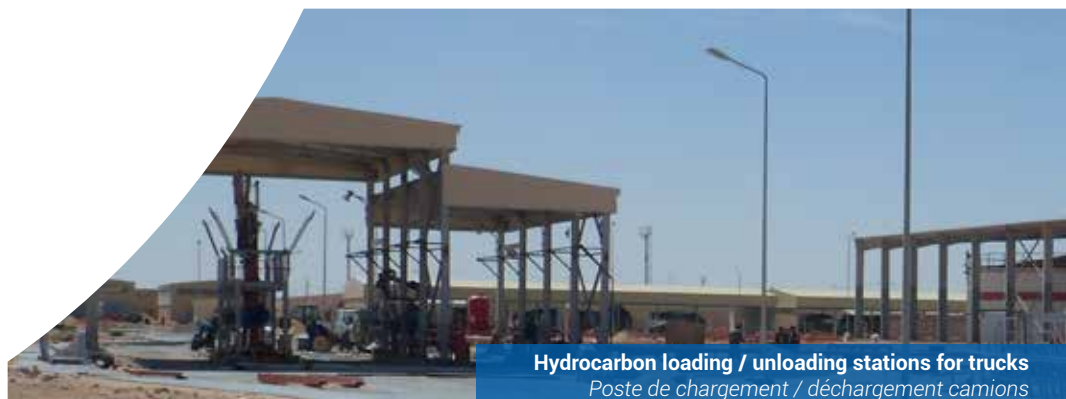
Loading station for trucks - Skid de chargement camions
