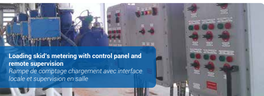
Loading station for trucks Skid de chargement camions dome
