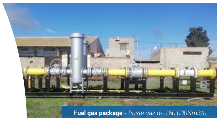
Gas station feeding a steel plant Station gaz 250 000 Nm 3 /h alimentant une aciérie
